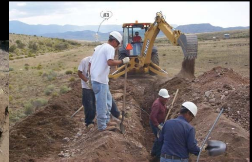
Fiber optic transmission
