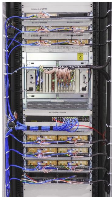
BPM Rack Front View
