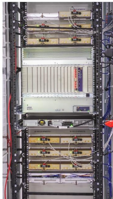
BPM Rack Rear view
